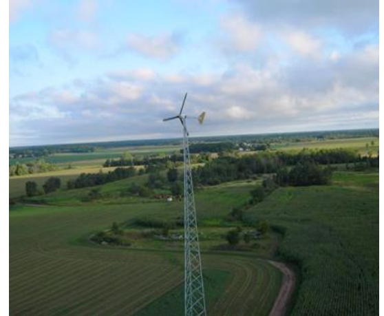
A Bergey Windpower 10 kW turbine installed on a Minnesota farm offsets the farm's energy usage and lowers operating costs.
