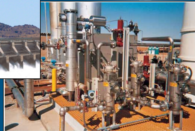
Methane gas digester system
